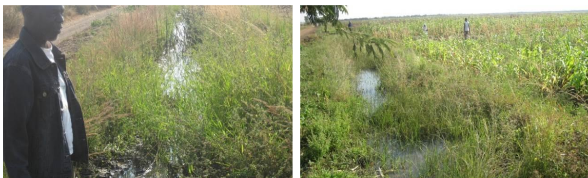
Figure 1. Shallow and grass choked canals at Tsvovani irrigation scheme
