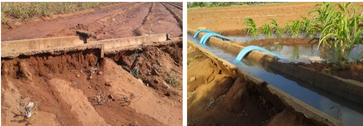
Figure 2. Eroded canal embankments in Vimbanayi and Mutorahuku irrigation schemes
