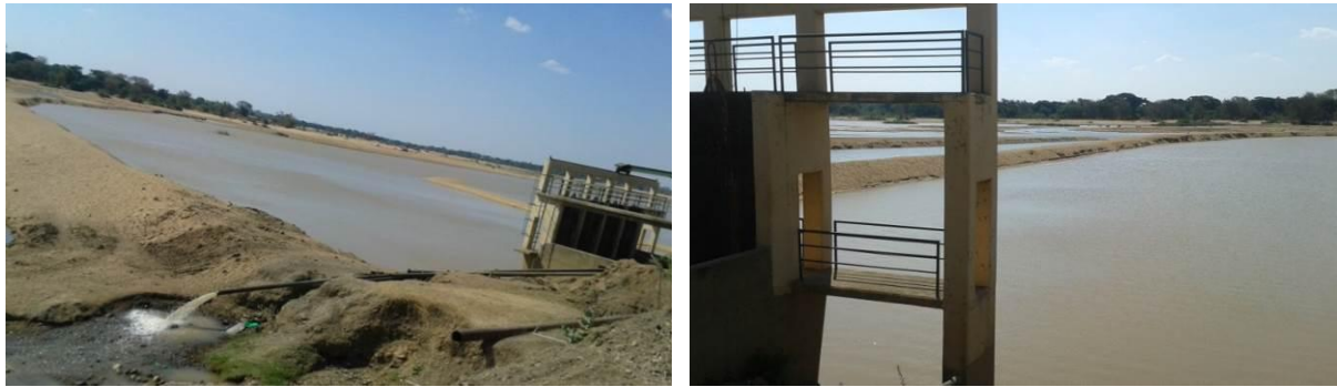
Figure 8. The Save River completely blocked at the Macdom pump house a week after the onset of the rainy season in November 2014
