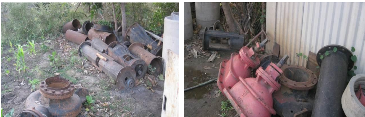
Figure 5. Part of the remains of the sand abstraction system equipment at Tsvovan
