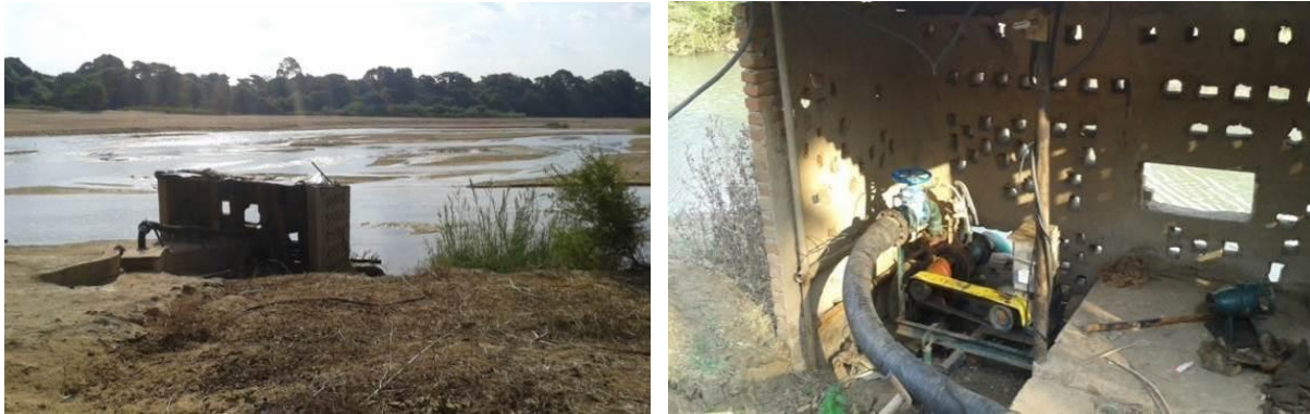
Figure 3. Pump plinth for Vimbanayi and Zuvarabuda constructed near the bank of Save River
