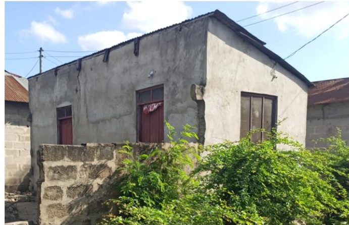
Figure 8. Exterior View of the Starter House Depicted in Figure 7 (Source: Field observations, 2021)
