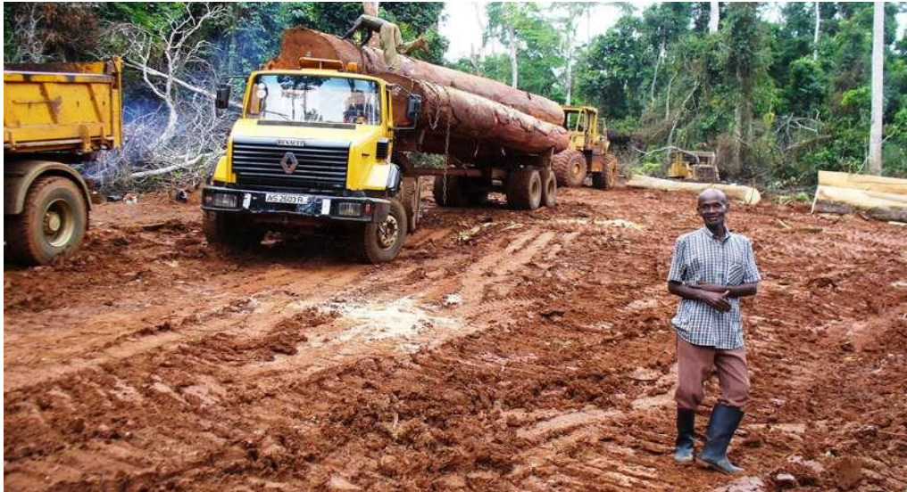
Figure 5. Wide area cleared by timber companies as their loading point (Photo: A legal logging operation in the Sui River Forest Reserve, Photo credit: Nicole Arcilla)
