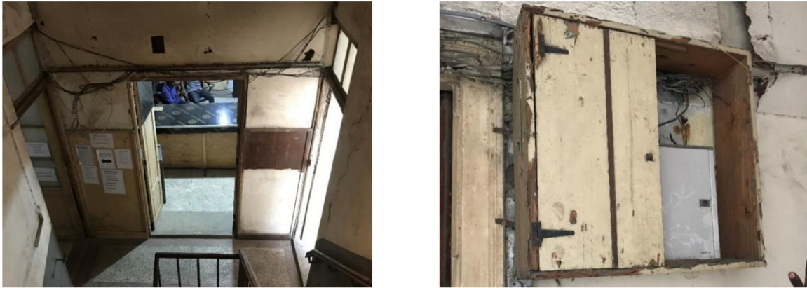
Figure 8. Old and poor electrical service system in the HOSCO building; Left: Exposed, spaghetti electrical wiring systems; Right: Old main switch/control panel (Source: Author, 2021)
